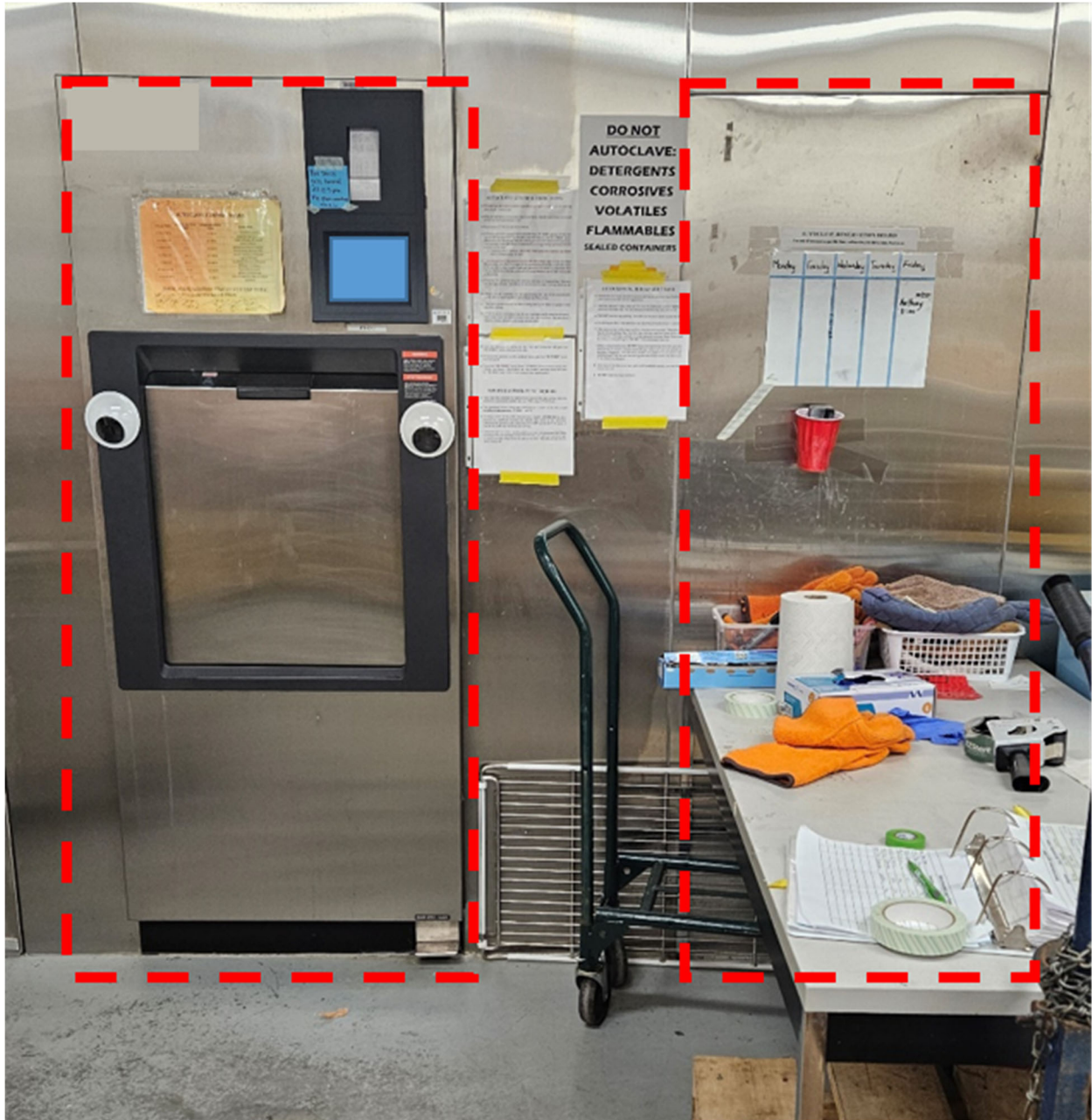
Figure 4. Placement of the two new autoclaves is available in the current wall.
