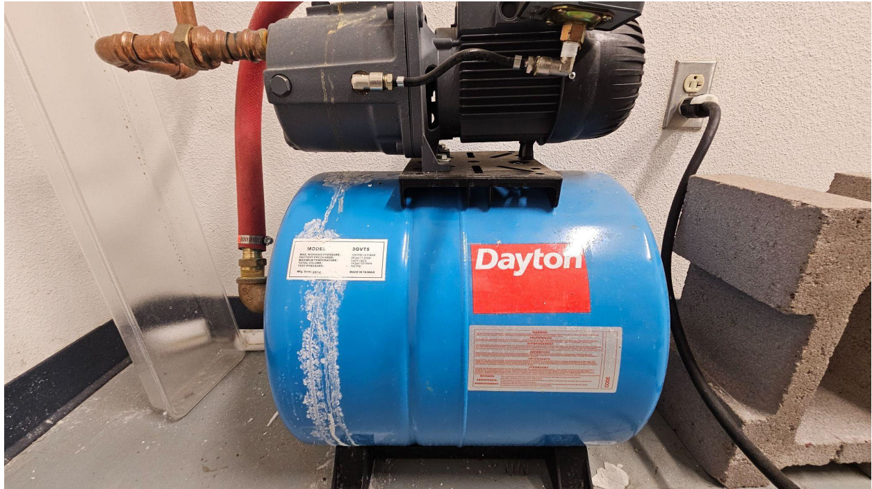
Figure 6. Pressure pump used to increase pressure for autoclave water supply.
