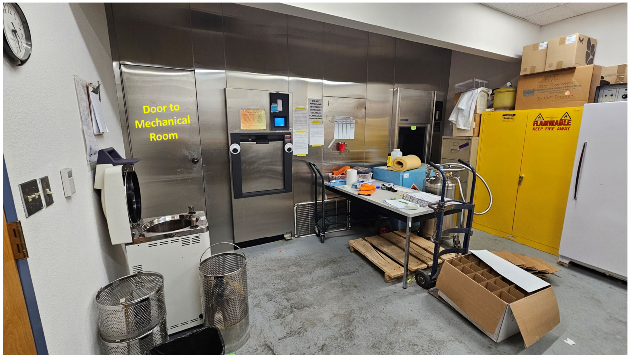
Figure 2. Instrument room. This room contains the control panel and access to the inner chamber of the autoclave.
