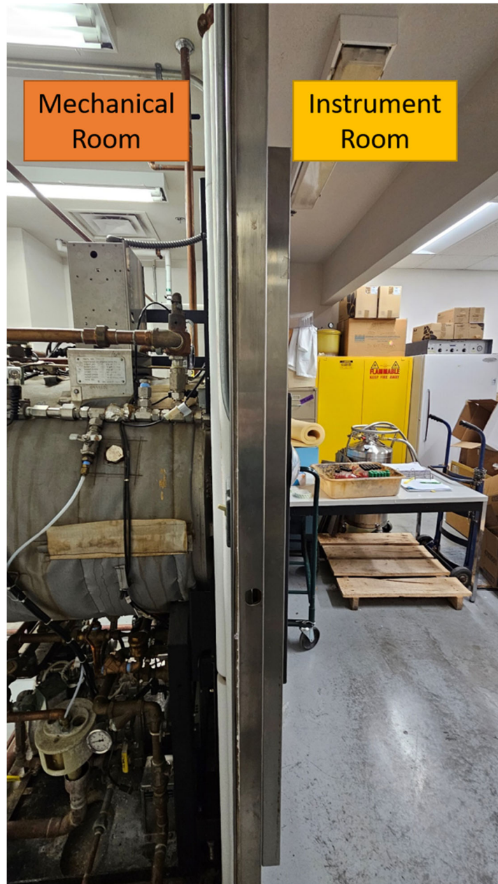
Figure 1. The autoclave room contains two parts: The mechanical room and the instrument room. A metal wall with a door separates these two rooms.
