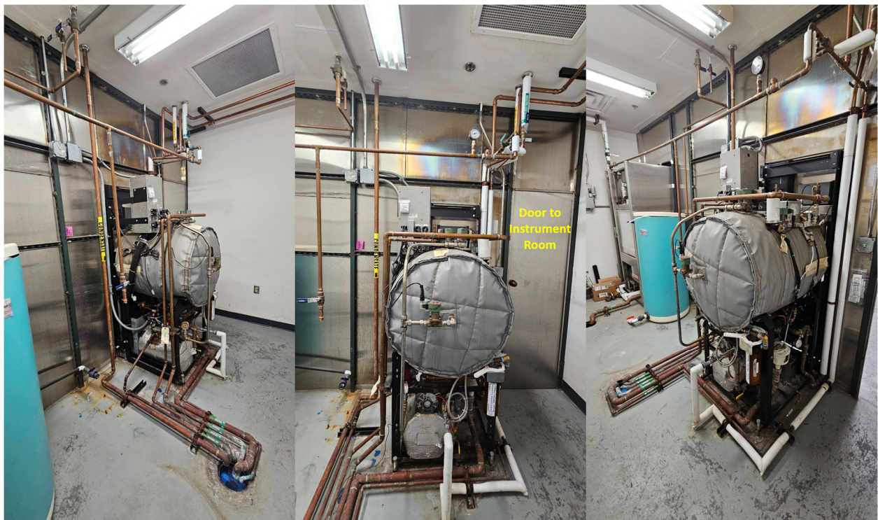
Figure 3. The mechanical room. This room contains the jacket, plumbing, and electrical hook ups for the instrument.
