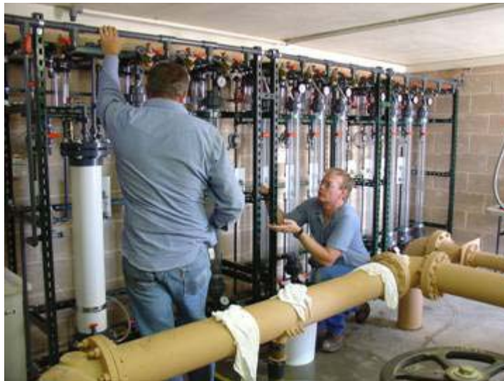
Figure A-1. Socorro Pilot Test Equipment.
