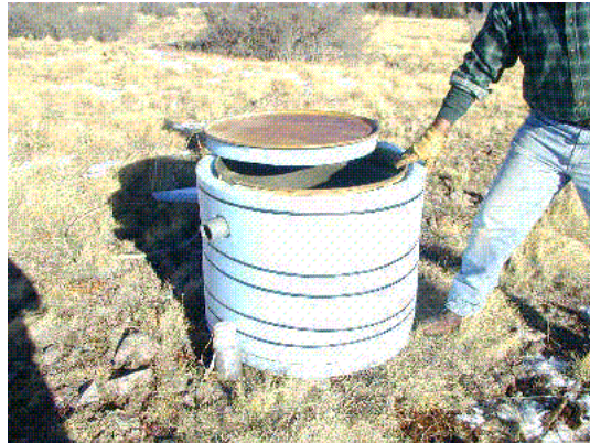
Figure 3.3: One of the four vaults hosting the seismometers is shown prior to shallow burial. Note that there is nothing particularly special about using steel cylinders to make the vaults rather than, say, a concrete box. However, old 55-gallon drums are handy almost everywhere and are commonly used in temporary deployments. The black, nearly horizontal straps secure the close-cell blue foam insulation to the outer surface of the cylinder. The short, narrow pipe protruding near the top of the vault provides an exit for the cabling. To ensure that the seismometer is thermally insulated on all sides, the bottom of the cap, shown sitting atop the vault, is also covered with a circular plate of blue foam. (Photo courtesy of Day Frostenson.)
