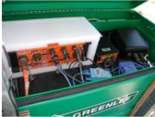
Figure 3.4: One of the four Greenlee vaults hosting the recording electronics. Clockwise from the top left: Q330 data acquisition system, Baler14 recorder, charge/load controller box, radio link, and ethernet switch. Batteries are kept in the box on which the electronics sit and are therefore not visible. Every vault was kept locked throughout the experiment to discourage vandalism. (Photo courtesy of Glen Gettemy.)
