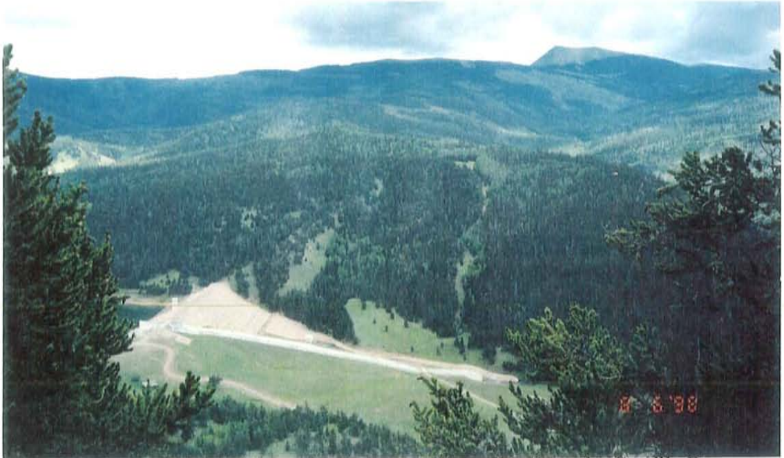
Figure 13 Outlet works slump located across the valley from the Costilla Dam Landslide. The landslide is outlined downstream from the dam by grass vegetation in the midst of the pine forest. Costilla Dam can be seen in this picture. The new spillway lies on top of the toe of the reactivated Costilla Dam landslide and stabilization berm.
