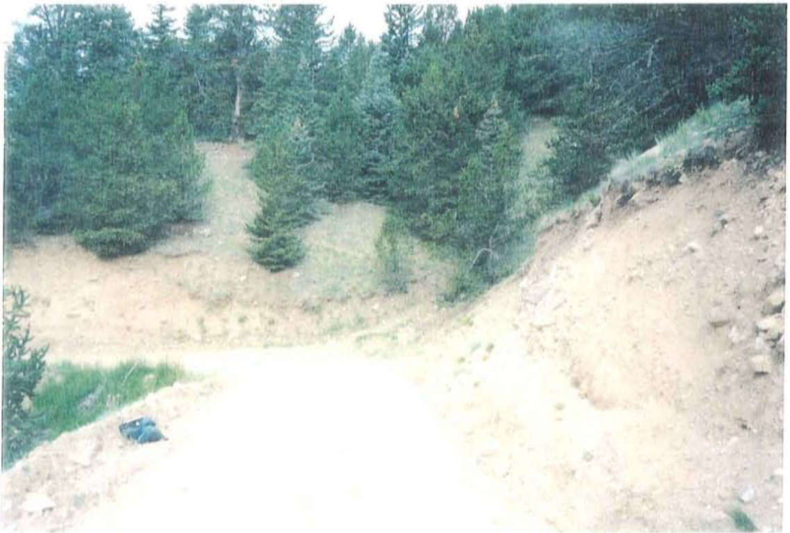
Figure 22 Gully defining lateral extent of Costilla Dam landslide complex. The gully located in the center of the picture is the northeastern lateral margin of the Costilla Dam landslide complex at the location of the star in figure 4. To the left of the gully when looking uphill is the landslide deposit photographed in figure 16, while to the right is the fluvial facies deposit of the Santa Fe Group photographed in figure 12.
