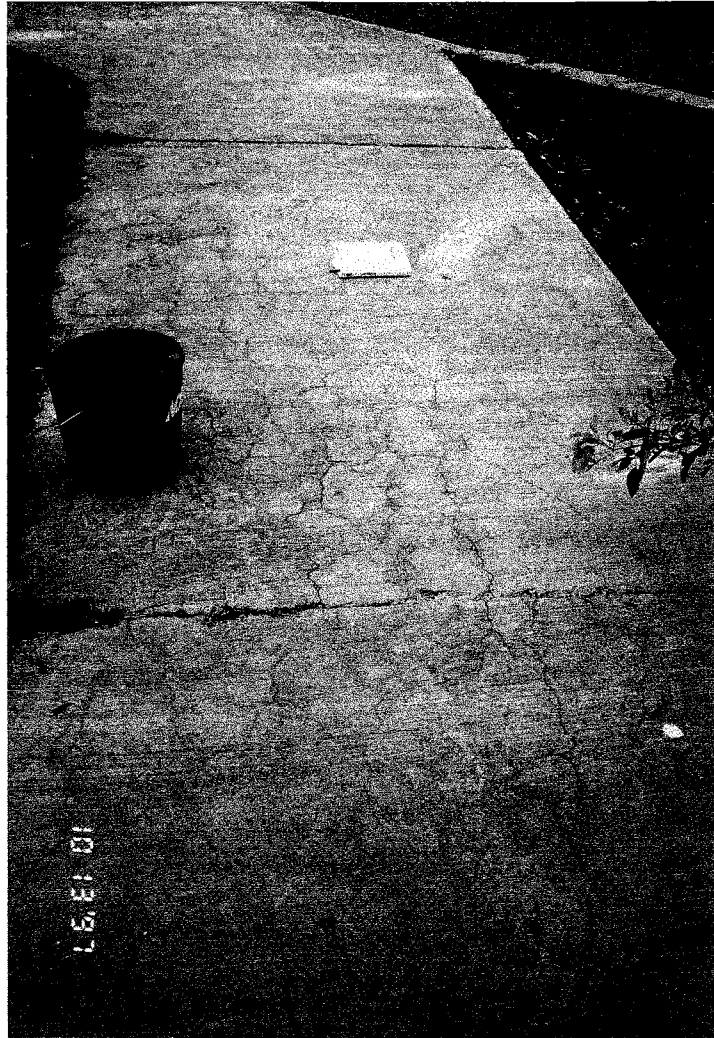
Figure 15. Map cracking on sidewalk where core sample 4 was taken. Core was taken near the yellow field notebook.
