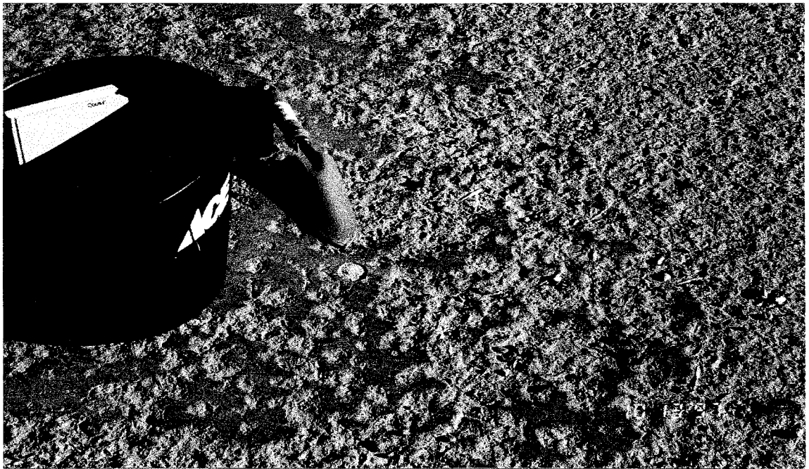
Figure 13. Popouts in sample area 11. Trowel is pointing to the core location.
