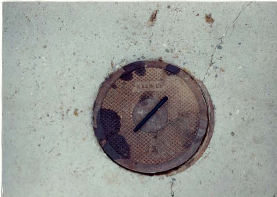
Figure 19 Photograph of UST refill cap cover (pen for scale is approximately 5 inches in length).
