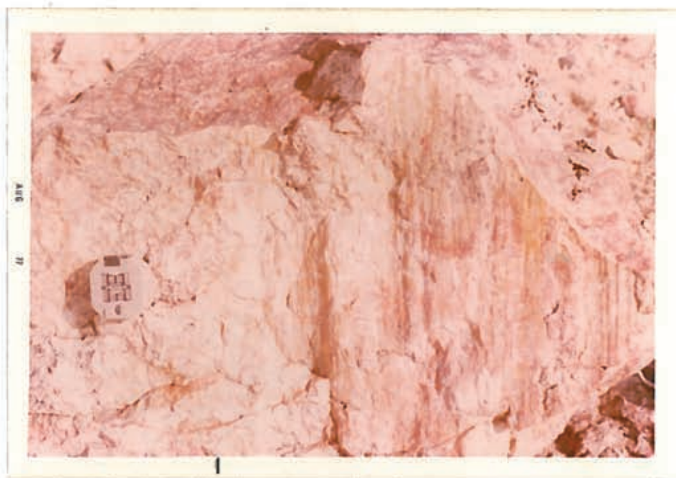
Figure 13. Slickensides on "joint" surface. (location--about 10 feet west of station 205)
