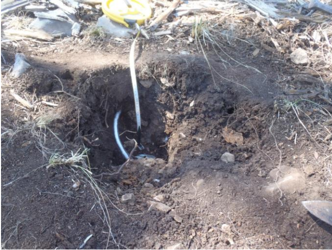
Figure 18: Photograph of RT 2 PCAPS installation.
