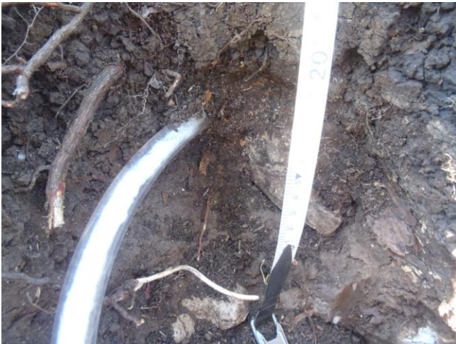
Figure 19: Close up photograph of RT 2 PCAPS installation.
